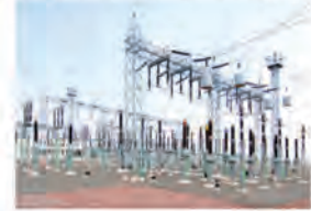
Structure and Transmission Line
